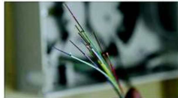
Fibre-optic cables carry services via Georgia to Armenia
